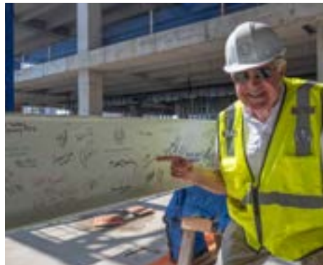
Novak points at the signed beam before it is placed at the topping out ceremony for Phase Two of the Capitol Complex Project.
