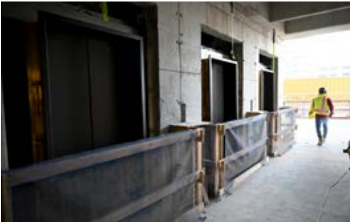
Unless the elevator crews are working at the opening of a hoist way and are tied off, the elevator hoist ways stay barricaded to prevent access. The only people allowed in the elevator corridor when the hoist way is open is the elevator crew. (Photo courtesy of TFC)
