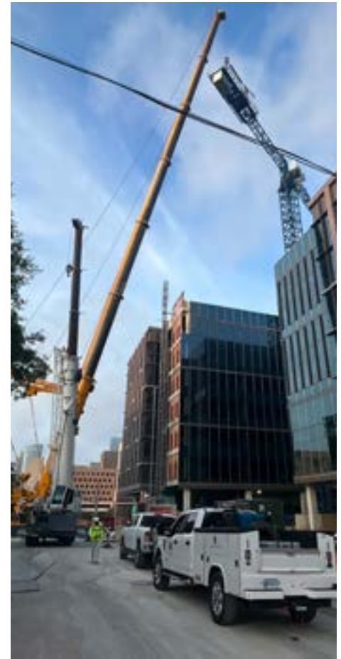
Above: The counterweight of the crane being hooked up and ready to fly to the ground. Bringing down a tower crane is a teeter-totter game of balancing. The crane is dismantled in an exact order to maintain the counterbalance and prevent the crane from tipping over. Crane pieces range in weight from 1,000 to 20,000 pounds. (Photo courtesy of JE Dunn)
