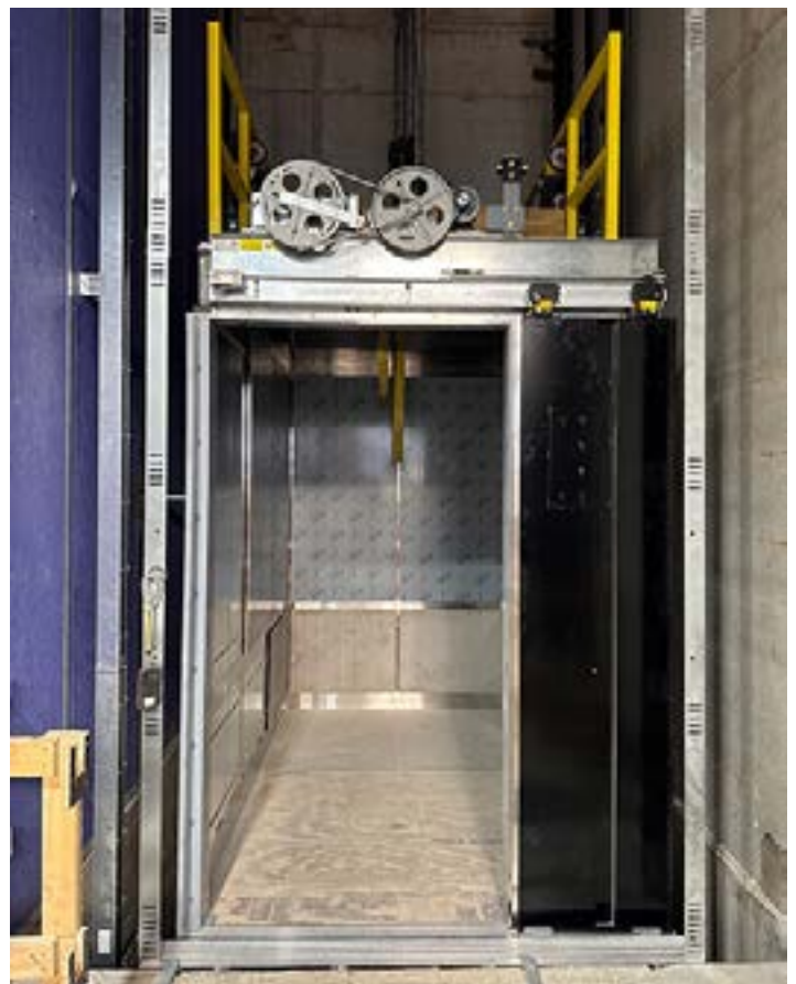
Top and Bottom Photos: Installation of the cab in the South 1 elevator in the 1501 Lavaca State Office Building. (Photos courtesy of K&M Elevator, LLC)
