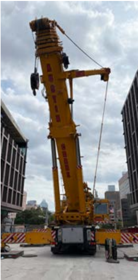
Above: An assembled 500-ton assist crane ready for work. The assist crane was used to dismantle the tower crane. While the assist crane was assembled, all the cables on the tower crane were disconnected, spooled, and secured. The process of dismantling the crane and removing it from a construction site takes three days. (Photo courtesy of JE Dunn)
