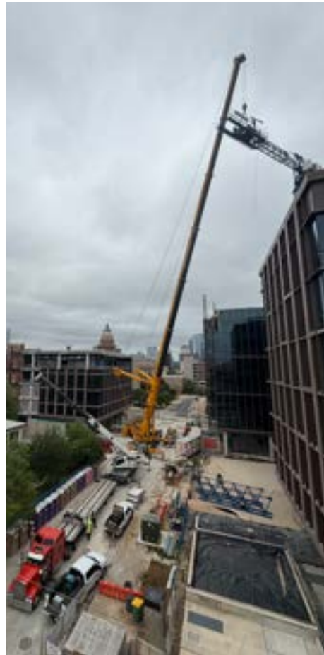
Above: Disconnected sections of the crane's jib lay on the ground. The mobile crane sits in front of the assist crane and loads the pieces onto trucks. It took sixteen semi-trucks to remove the crane from the 1501 Lavaca project site. As soon as the trucks were loaded, the in-demand tower crane was taken to another construction site for assembly. (Photo courtesy of JE Dunn)
