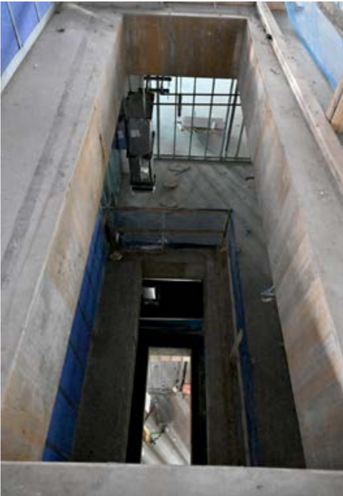
View looking downward into an elevator hoist way. (Photo courtesy of TFC)
